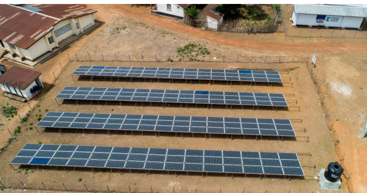
Solar off grid system with NEF logo in the background, Gbinty Town, Port Loko District, Sierra Leone (COOPI)
