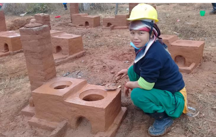
Renewable World: Training of the technicians to construct and market one of the three types of improved cookstoves as part of the E4H project.
